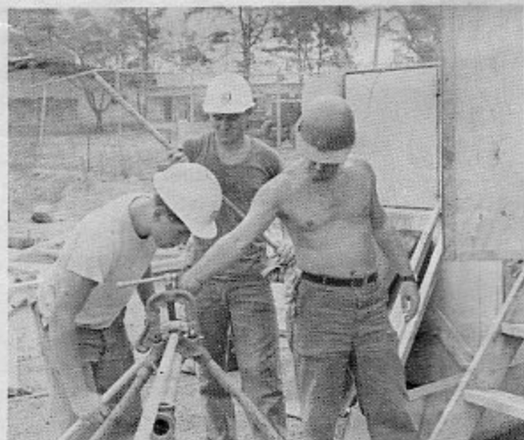
P.D. MAZIEKA UTP3, J.W. JENKINS UT3, C.T. TIBBS UTP2 THREADING PIPE AT III MAF BARRACKS PROJECT.
