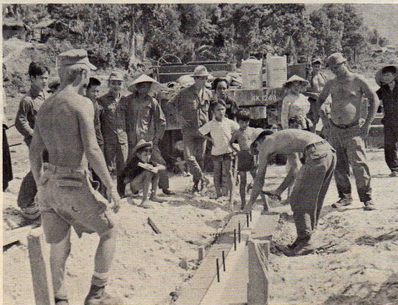
DETACHMENT FROM MCB-53, BEGINNING CONSTRUCTION OF BRIDGE AT TRA BONG, SOUTH OF DANANG.
