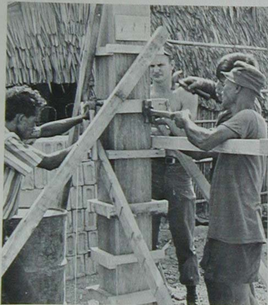
BU2 Danny G. Smith (behind column) from Brookhaven, Mississippi, shows trainees how to set up the form for a concrete column. Made up of war refugees and former Viet Cong, the trainees are learning the skills that will help them rebuild South Vietnam.
