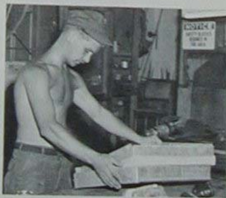
SW2 Leon Kowalski from Detroit, Michigan, fabricates a flexible connection at Bravo Company shops.
