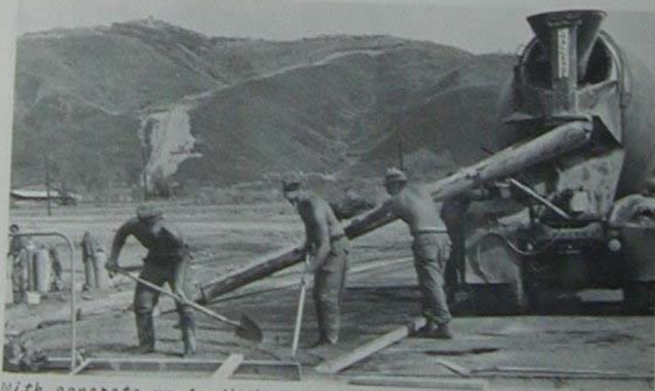
With concrete up to their knees two builders lay the slab for a butler building while a TM driver guides the flow from his truck.
