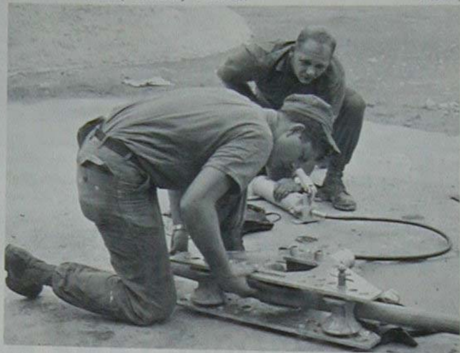
CE2 James Scruggs (left) from Wadley, Georgia, and CECN Kenneth Hubbs from Phoenix, Arizona, bend two inch conduit for the electrical system of the new automatic concrete batch plant operated by Alfa Company.
