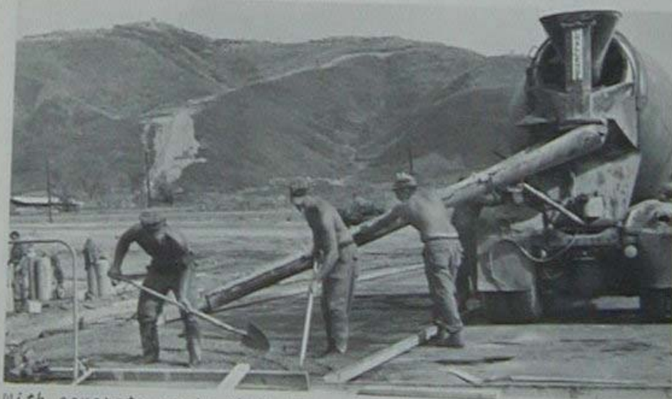
With concrete up to their knees two builders lay the slab for a butler building while a TM driver guides the flow from his truck.
