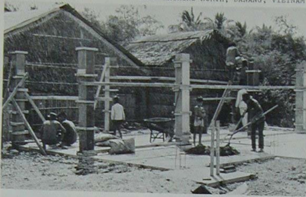
Builder trainees of Seabee Team 5301 pour columns at Phe Me village in the province of Ba Xuyen. The columns are part of the now completed village headquarters building.
