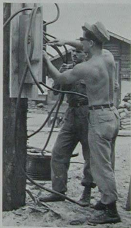
CE2 Gary Welles (right) from Wildesbarre, Pennsylvania, and CE3 Bruce Reese from McKeesport, Pennsylvania, install emergency switches to the Administrative area.
